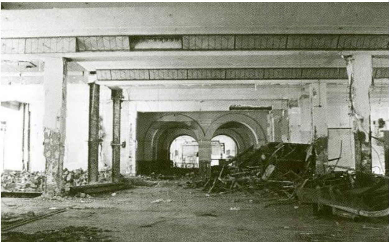
Figure 64 – The degraded ground floor in 1984 with Art Deco style light fittings, only the remnant arches in the background remained from the original presentation
