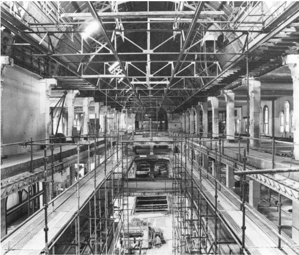
Figure 69 – The concrete slabs were removed by 1985 and the interior voids recaptured, note the extent of original interior fabric
